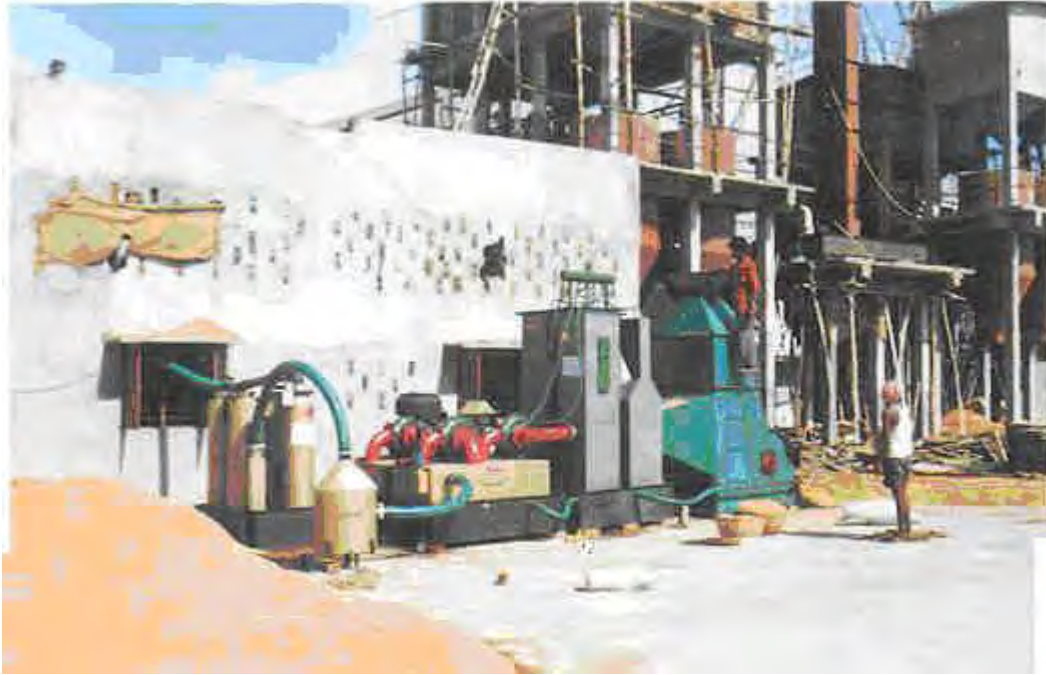
a 100KW capacity Rice-Husk based Gasifier installed in a rice mill in Andhra Pradesh
