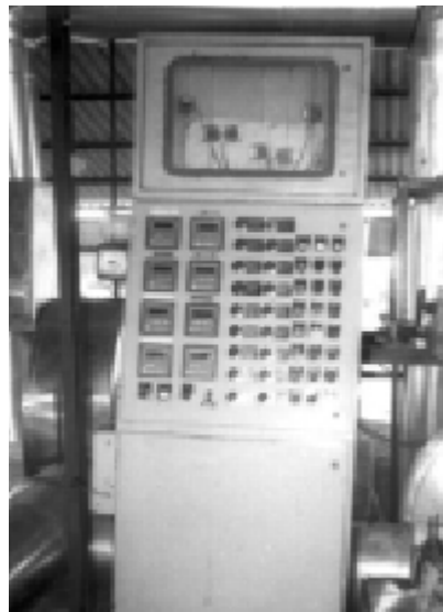
Figure 2. Programmable Logic Controller (PLC)-based control System
