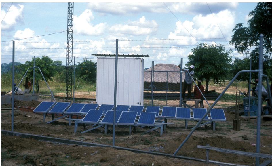
Solar panels, Pemba-Metuge, Maputo, Mozambique ©UN-Habitat/Ricardo Rangel
