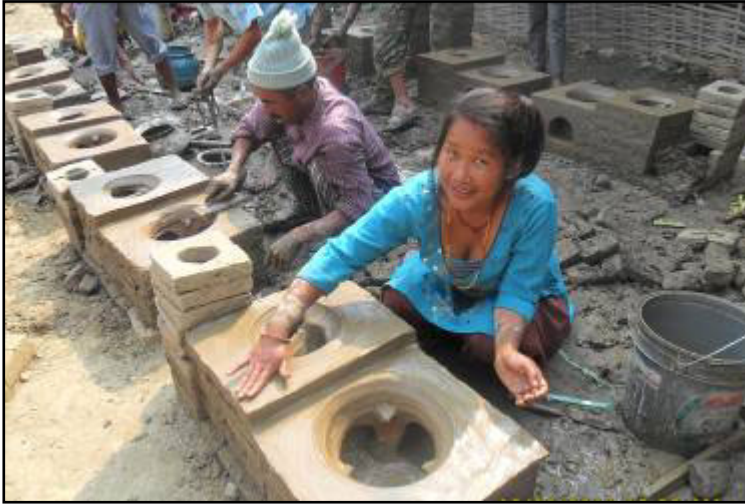
PHOTOGRAPHER: Bhagirath Prasad Ghimire TITLE: Building mud stoves for efficient cooking CDM PROJECT: 4530 Efficient Fuel Wood Cooking Stoves Project in Foothills and Plains of Central Region of Nepal COUNTRY: Nepal
