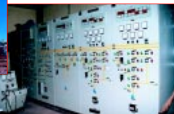
View of control room - generator panels
