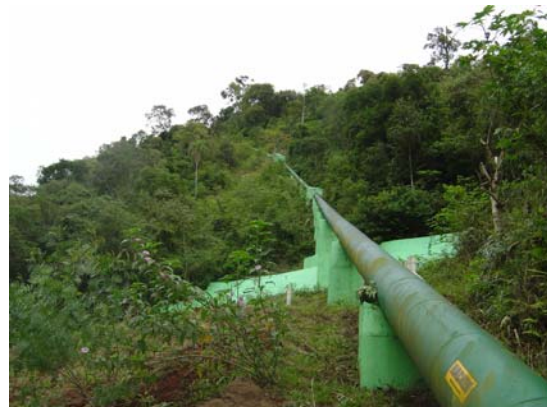
Figure – Creral waterfall pipeline
