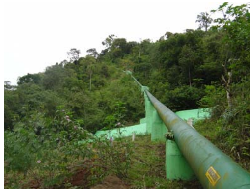
Figure – Creal waterfall pipeline
