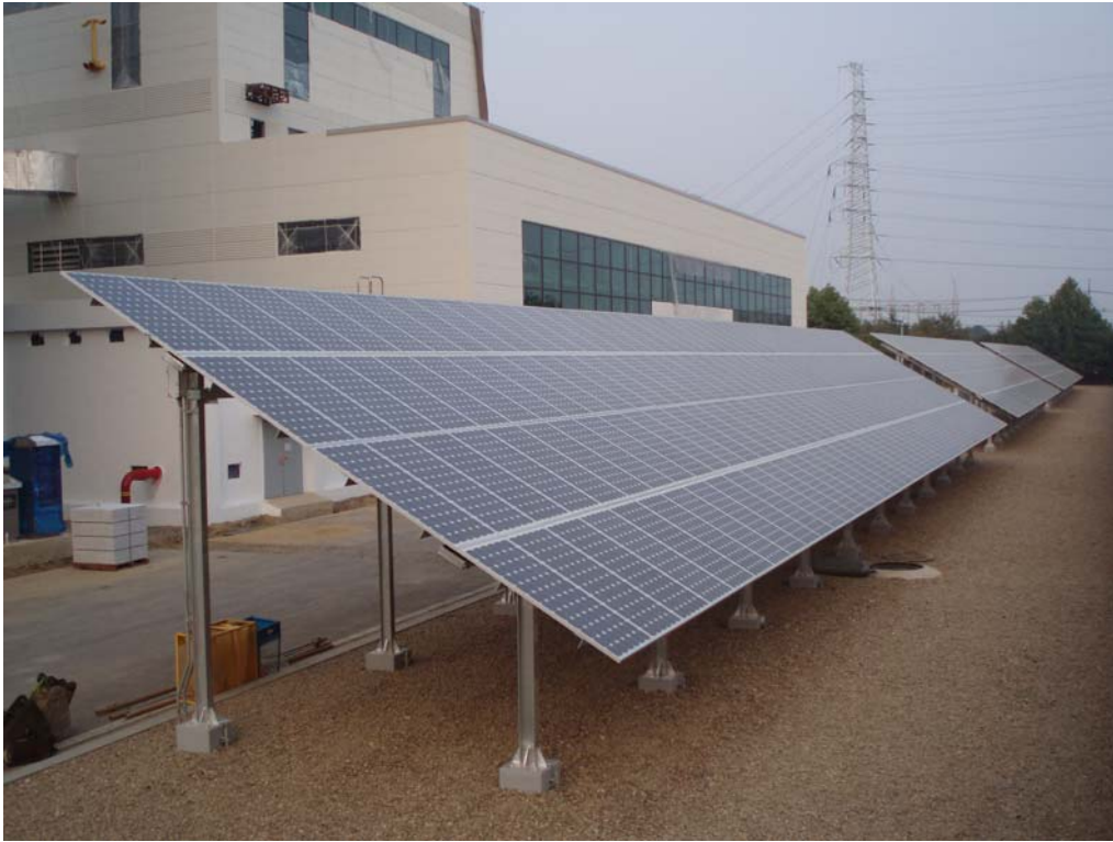
<Figure 2> Daegu PV Power Plant
