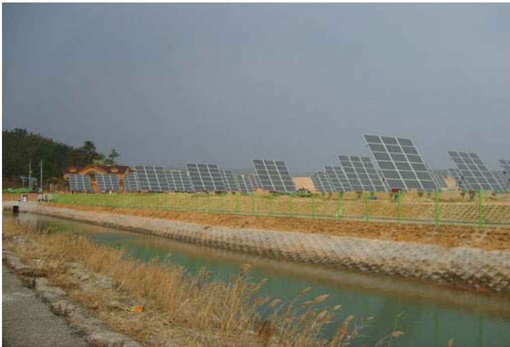
<Figure 3> SinanJeungdo PV Power Plant
