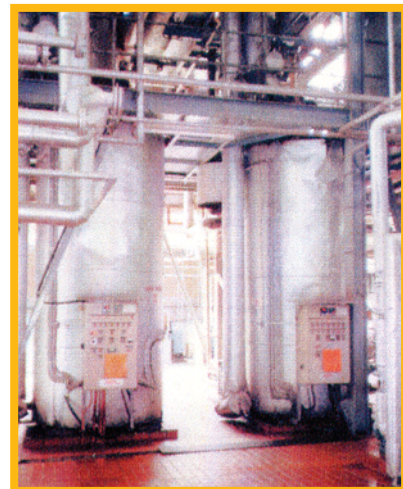
Plate 2 : High Pressure Steam boilers Fired by biogas
