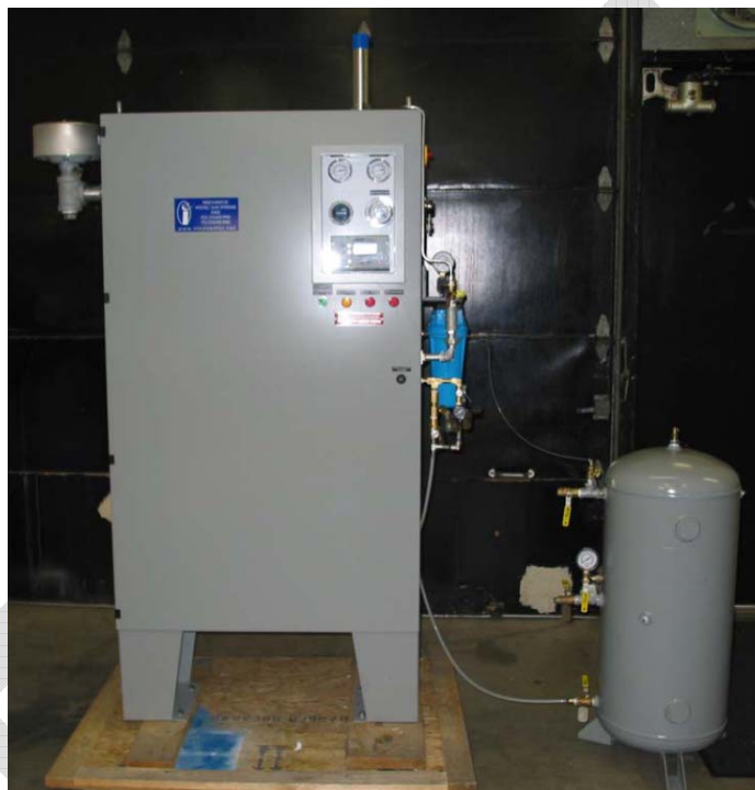
Figure 25: Nitrogen generator with a buffer tank
