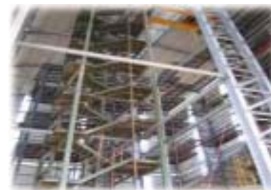
Babcock & Wilcox Volund Boiler structure & platform
