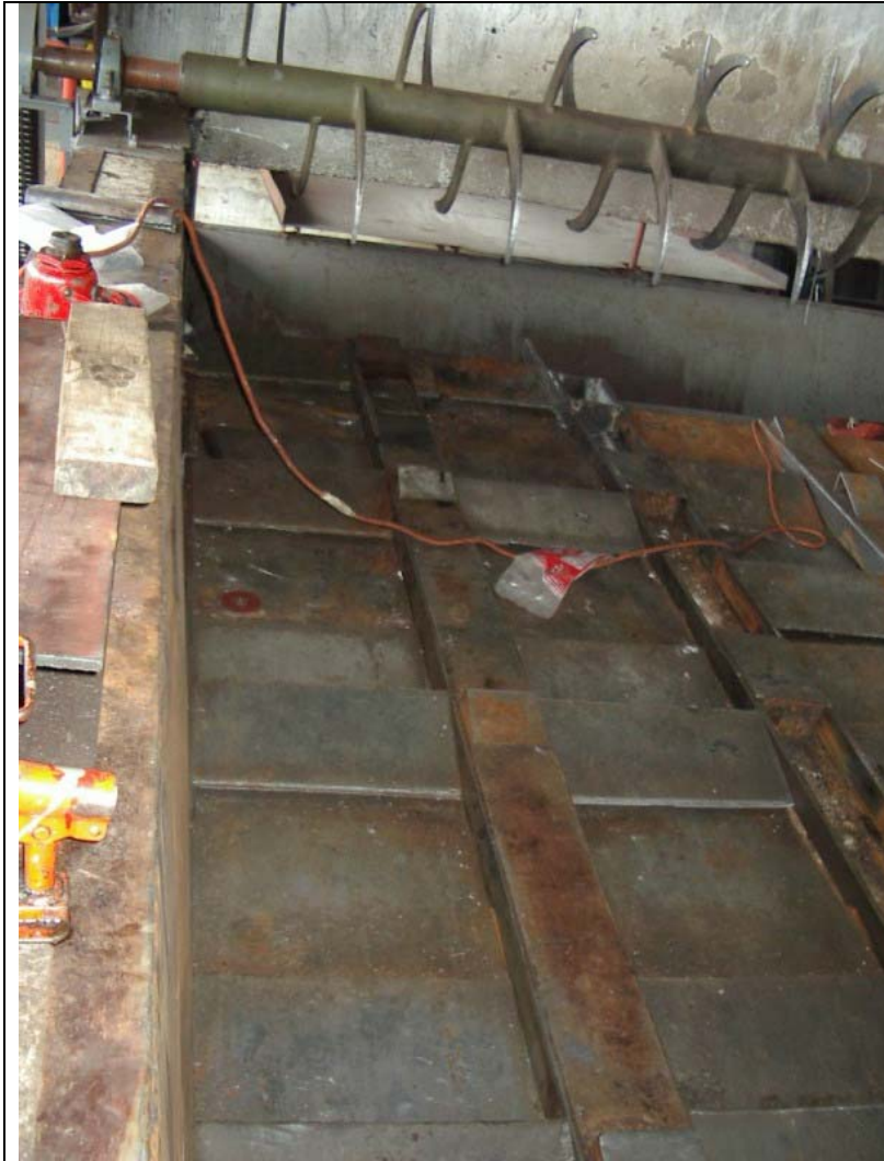
Figure 11: Moving floor damaged due to wrong design and excessive wear and tear – repair works being carried out
