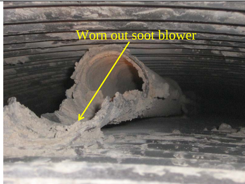
Figure 15: Damaged soot blower
