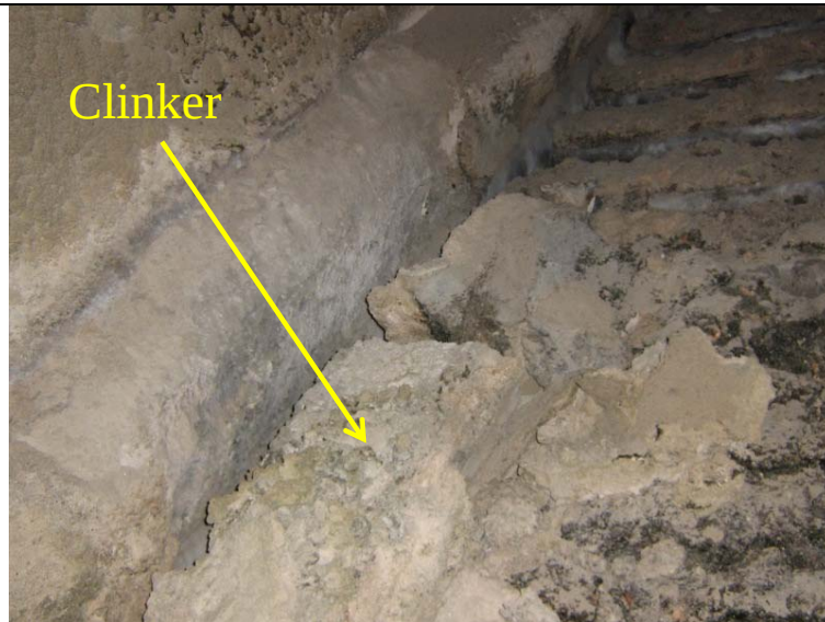
Figure 5: Excessive clinker formation on furnace floor (step
