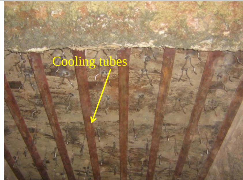
Figure 8: Repair underway for damaged furnace ceiling. Water cooled coils are exposed when refractory is damaged causing excessive corrosion of water coils to take place
