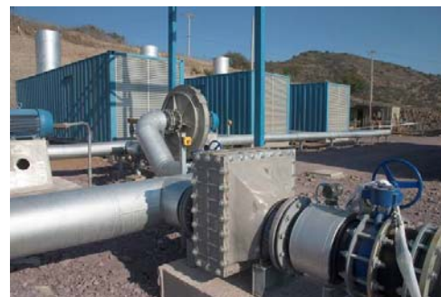
Figure 1.3 Principal valve, flame arrester, blower
