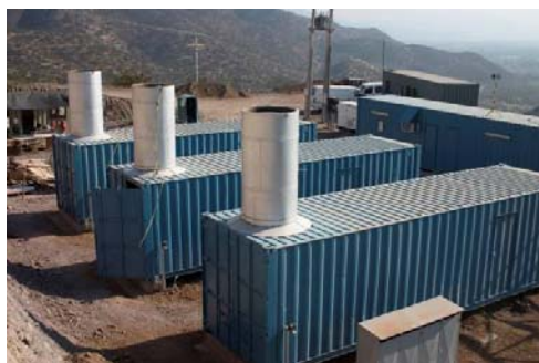
Figure 1.2 Flaring station general view
