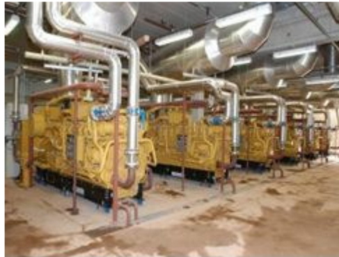
Figure 1.5. Generators used to produce electricity
