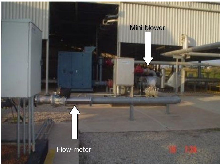
View of the mini-blower, indicating the flow-meter.
