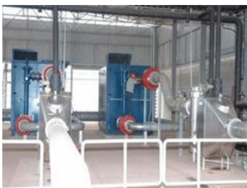
Figure 1.3. Compressors (blue) and dryers (metal)
