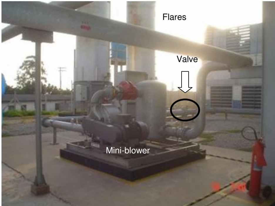
View of the mini-blower, indicating the flares and one of the valves.
