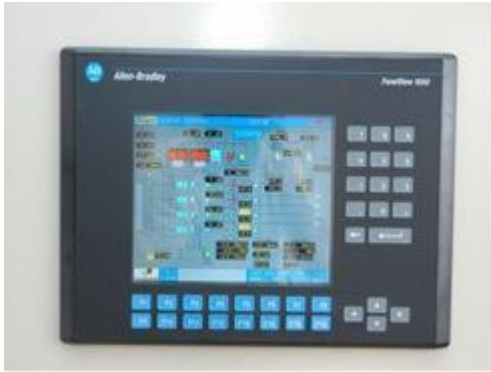
Figure 1.7. PLC Controlling System panel
