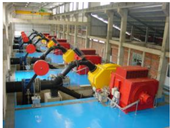
Picture 2: Turbines & Generators (5 Units)
