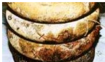
Tubes with nitrate induced SCC in a waste heat recovery boiler
