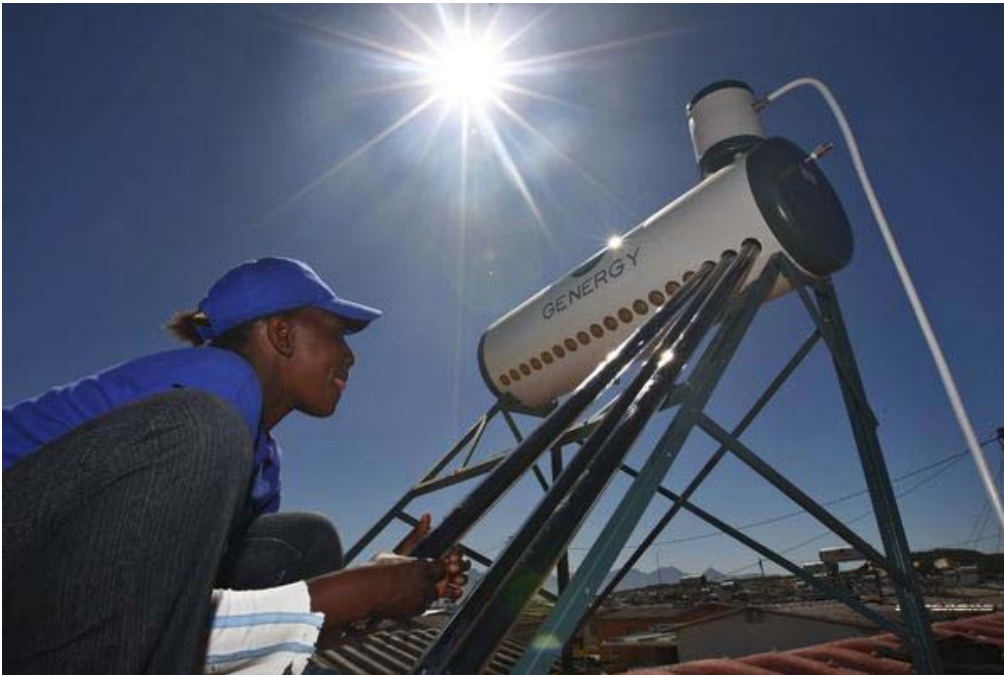
Catching the sun. Clean Development Mechanism (CDM) project 0079 – Kuyasa low-cost urban housing energy upgrade project, Khayelitsha, Cape Town, South Africa. Under the CDM, projects that reduce greenhouse gas emissions and contribute to sustainable development can earn valuable, saleable credits. Photographer: Nic Bothma.
